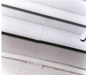
Asbestos lagging on pipe
